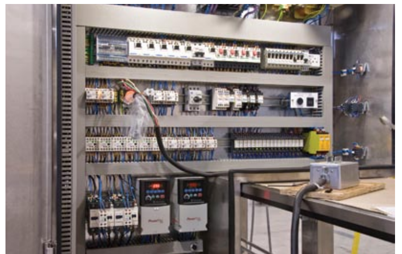
Known for its control panel manufacturing skills, this Newmapak version features Festo and Schneider Electric components operating a servo-driven high-speed capping machine that synchronizes the capping heads with the bottles to maintain optimal capping torque.
